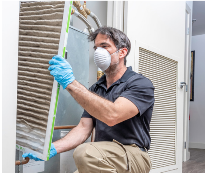
In many cases, HVAC systems degrade over time. This is why it is vital to begin any HVAC project with an assessment. (Source: RenewAire)
