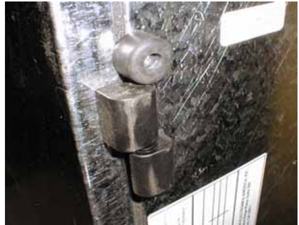
Figure 7. Rubber Door Keeper installed on Blower Access (large)
