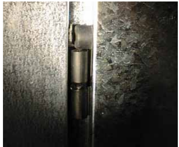
Figure 8. Rubber Door Keeper installed on Filter Access (small)
