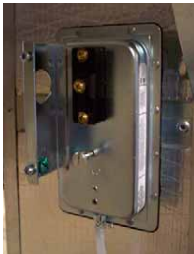
Switch with cover plate removed. Always reinstall cover plate.
