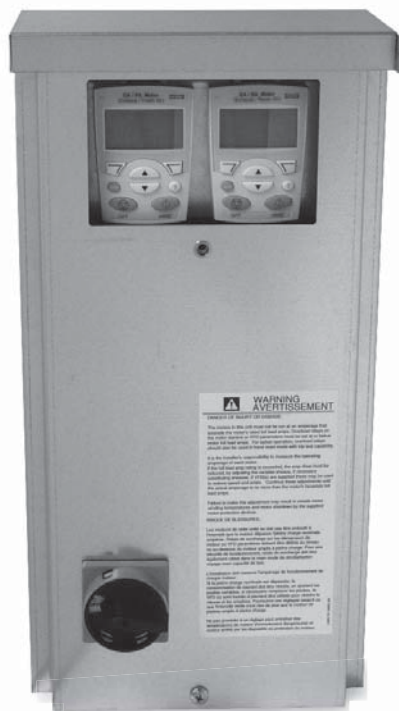
VFD KEYPADS IN E-BOX
