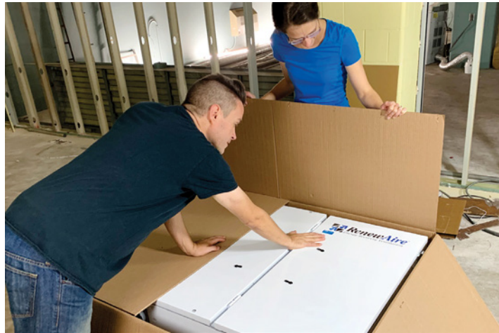
Bunker homeowner Ruben Romero, along with his wife, prepare to install their RenewAire EV450 ERV.
