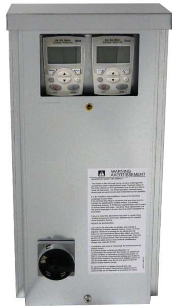
FIGURE 16.5.1 VFD KEYPADS IN EBOX
