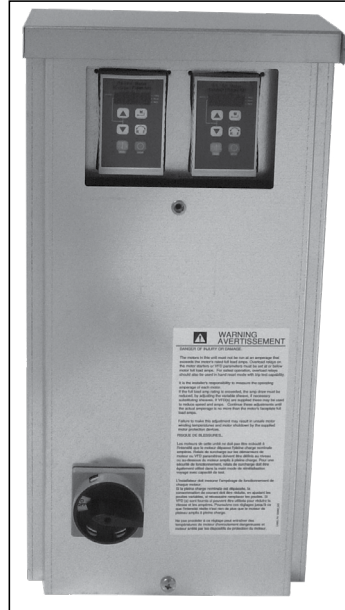
FIGURE 16.5.5 VFD KEYPADS IN EBOX
