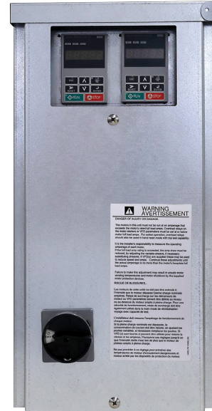
FIGURE 15.6.9 VFD KEYPADS IN EBOX
